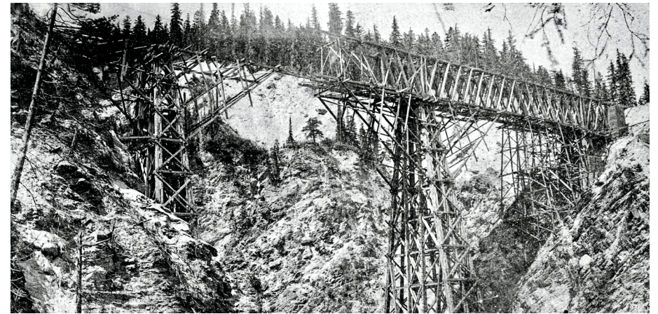
Buell also took this view of the Stoney Creek bridge as it neared completion in early August 1885. Note the bracing beneath the bridge chords, and the gap in the centre of the span. Construction of this remarkable structure required only five weeks and three days during a seven-week period, in which eleven work days were lost due to weather and the deaths of two workers.
