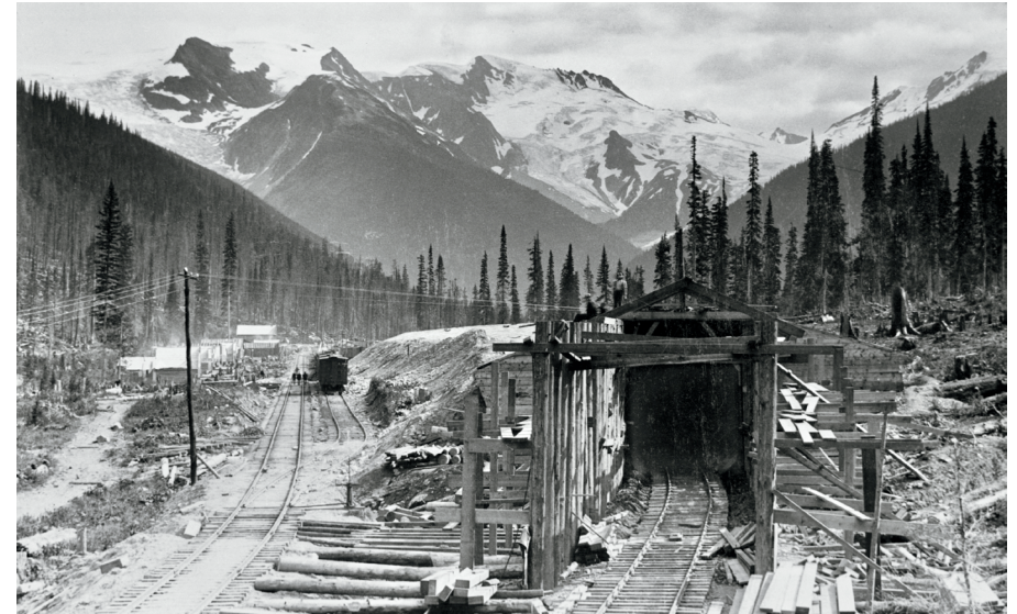
At 3,098 feet, 17 Shed was initially the longest in Rogers Pass and on the CPR. It was under construction when William Notman took this photograph in the summer of 1886, either standing atop a rail car or on the roof of 16 Shed. Most of 17 Shed had already been buried to strengthen it. You can see the shed curving to the left in the mid-background. Summer track is to the left of the shed. The construction tote road is on the extreme left. Today's Trans-Canada Highway roughly follows the tote road's route. The first Rogers Pass station is in the background on the left.
